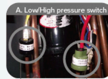
Low pressure switch High pressure switch
