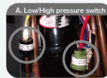
Low pressure switch High pressure switch
